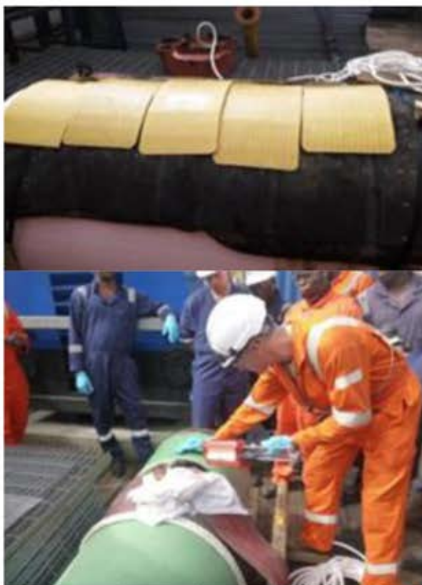
Composite plate manufacture on the foot print of the dented area & primer application (training picture). ●
