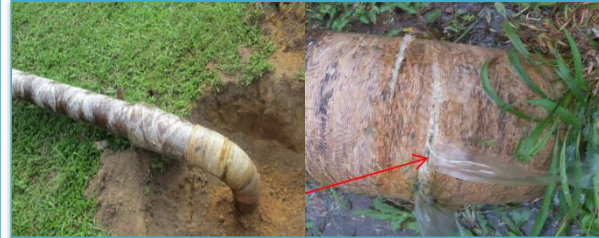
View of the elbow and leak point prior repair
